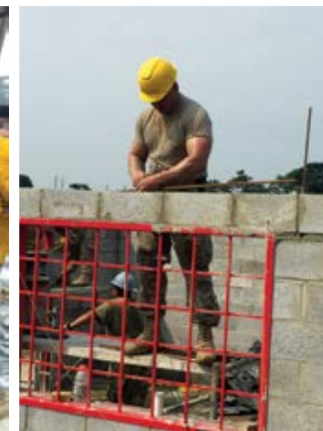
Master Sgt. Garrad Johnston, 489th BSB, helps build walls for a health clinic at San Pablo, Guatemala.
