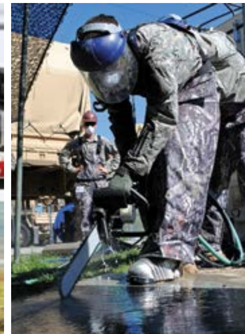
Spc. Kevin Gwilliam from the 624th Engineer Company, 1457 Engineer Battalion, uses a wet saw to cut a section of concrete as part of a renovation project on a restroom facility at the Renegade Point Marina, Strawberry Reservoir, June 8.
