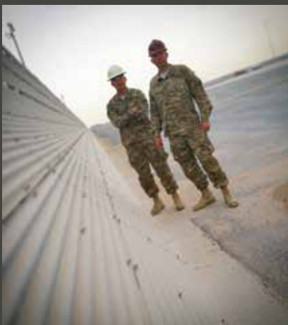
The 577th Expeditionary Prime BEEF Squadron Commander, Lt. Col. Paul Waite and Senior Master Sgt. Carl Greene, first sergeant pause after reviewing the progress on a project to modify an airfield-taxi way at Al Udeid AB, Qatar.
