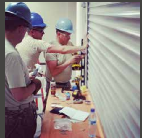
Tech. Sgt. Jared Webb, 577th Expeditionary Prime BEEF Squadron structures lead, installing a roll-up door as Airman 1st Class Casey Weldon and Lt. Col. Paul Waite, 577th EPBS commander, watches while deployed to an undisclosed location in Southwest Asia.
